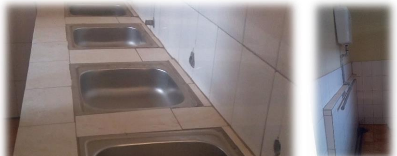
Clean Sinks and toilets at Lumakanda Police Station
