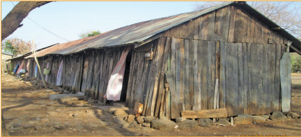
Dilapidated police housing at Isiolo Police Station in Isiolo County
