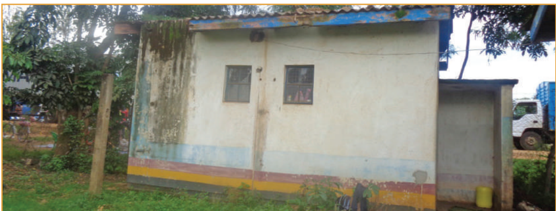
A toilet which was converted into a house in Malaba Police Station. It accommodated two officers.
