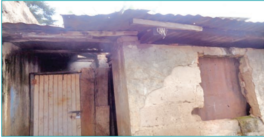
A dilapidated officer's housing at Mbale Police station in Vihiga County (Source: IPOA, 2014)
