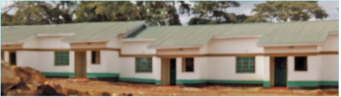
IPOA Photo: Incomplete modern houses for officers at Matunda Police Station which were constructed through the support of the County Government of Kakamega but have caused divergent opinion between the County Government and the National Government.
