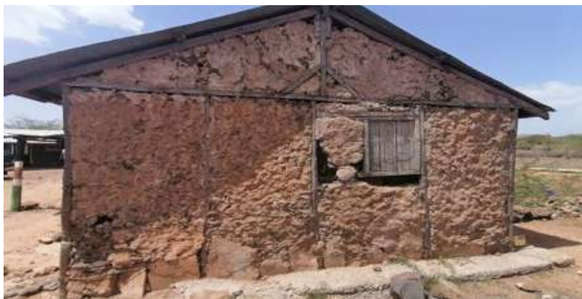
Photo 1: A dilapidated and insecure structure at Loglogo Police Station
