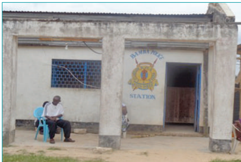
Bamba Police Station lacking a roof
