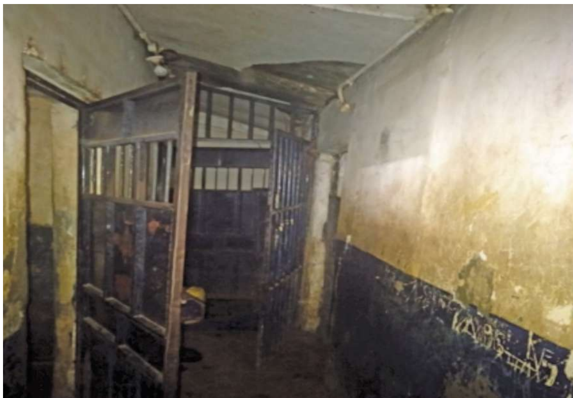
Photo 1: Cells in a deplorable condition at Wanguru Police station
